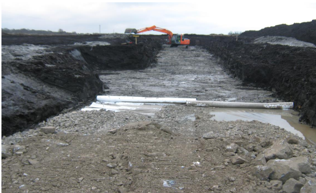
Typical road deep road detail with large boulders used as starter layer.
